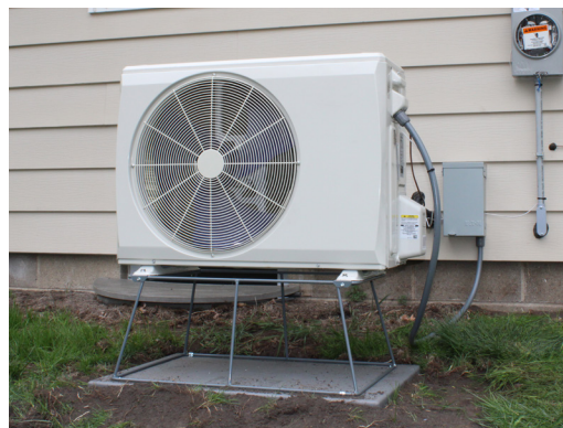
Equipment stand: keeping the unit above the snow (to some degree).
